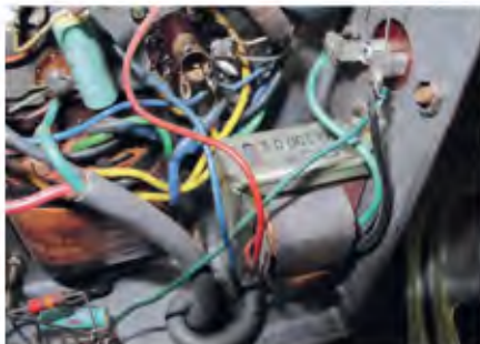
Fig.6: the output transformer had the date 30 October 1968 stamped on it.
