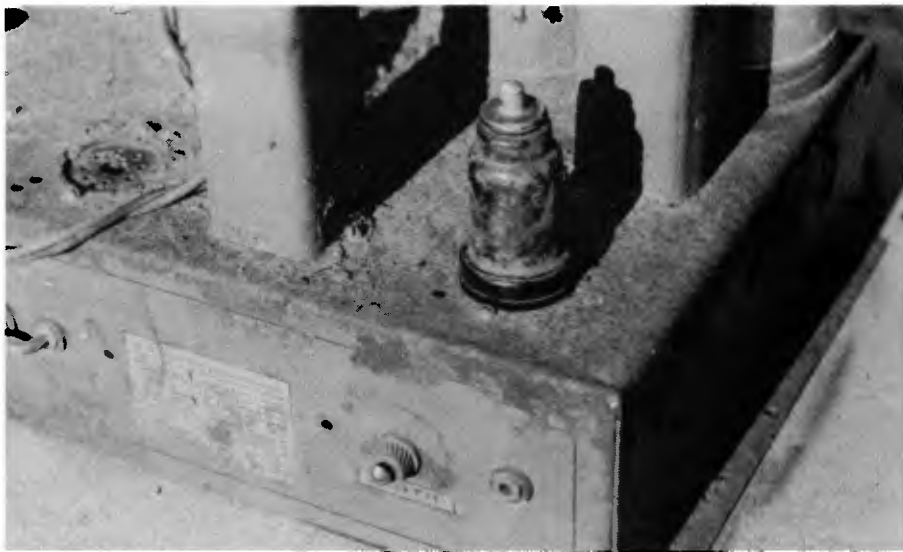
A badly rusted chassis requires anti-rust treatment before repainting. Failure to prepare the chassis properly prior to painting will result in the rust quickly breaking through the new paintwork.
