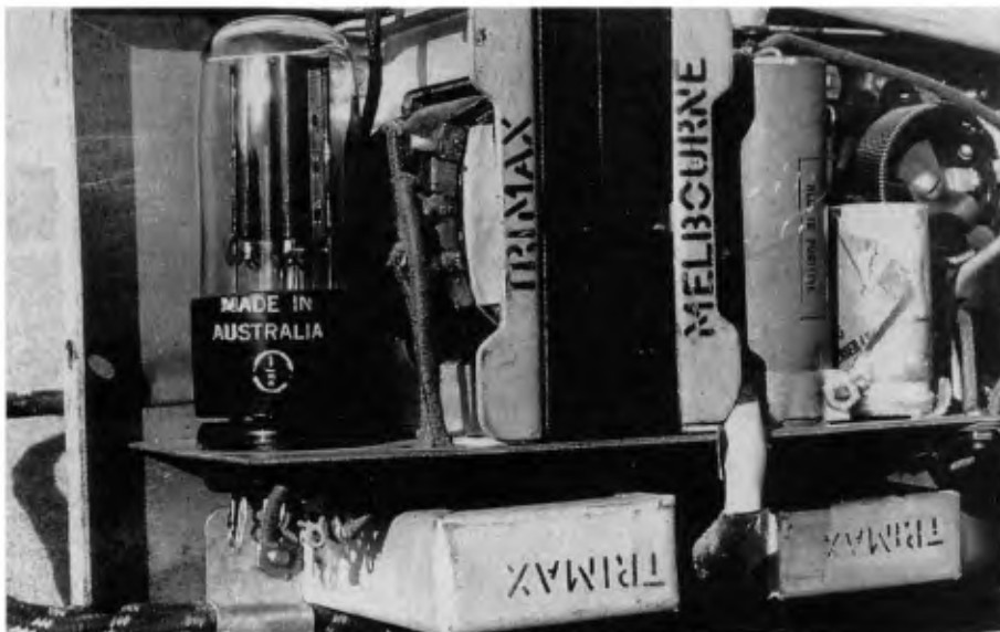
This view shows the power transformer, the 5Y3GT HT rectifier and the two Trimax brand filter chokes (beneath the chassis).
