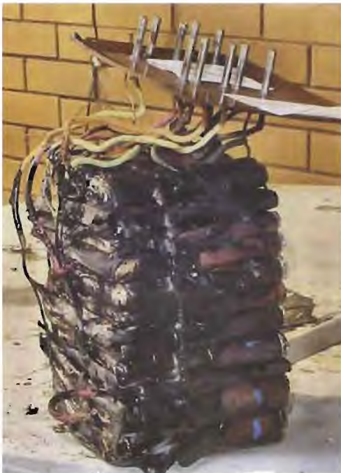
The plug-in capacitor box contained a large number of faulty paper capacitors, which meant that a complete new assembly had to be made up.
