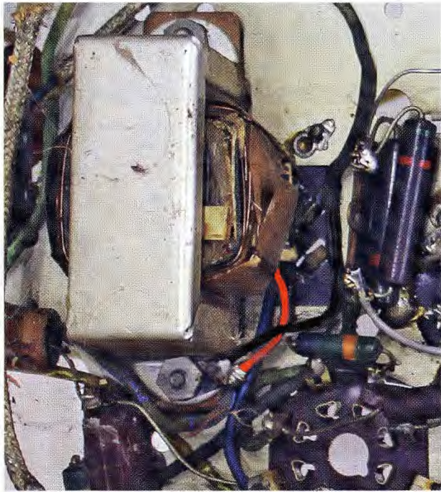
A particular problem in this set is that the HT from the rectifier and the secondary of the output transformer were connected to its frame, which was insulated from the chassis. This particular set also had excessive HT of 329V which caused occasional arcing between the output transformer primary and the earthed secondary.
