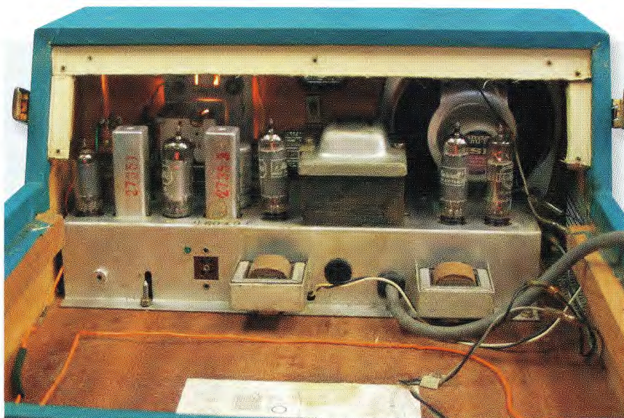
The chassis is crammed into the front of the case and the two audio out transformers hang off the rear. The orange wire is the aerial loop.
