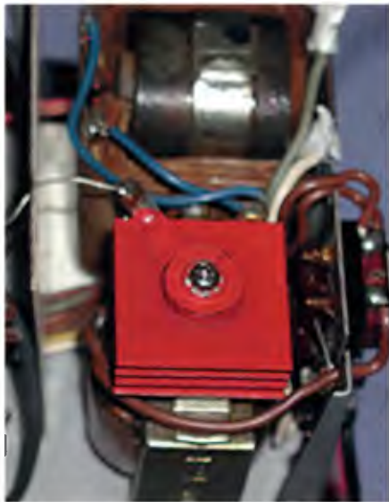
◀ Fig.2: selenium rectifier stacks are famous for producing lots of toxic fumes when they fail. That's why many people prefer to replace them with modern rectifiers. Still, you have to be careful because modern rectifiers can lead to much higher surge currents and have lower forward voltages.
